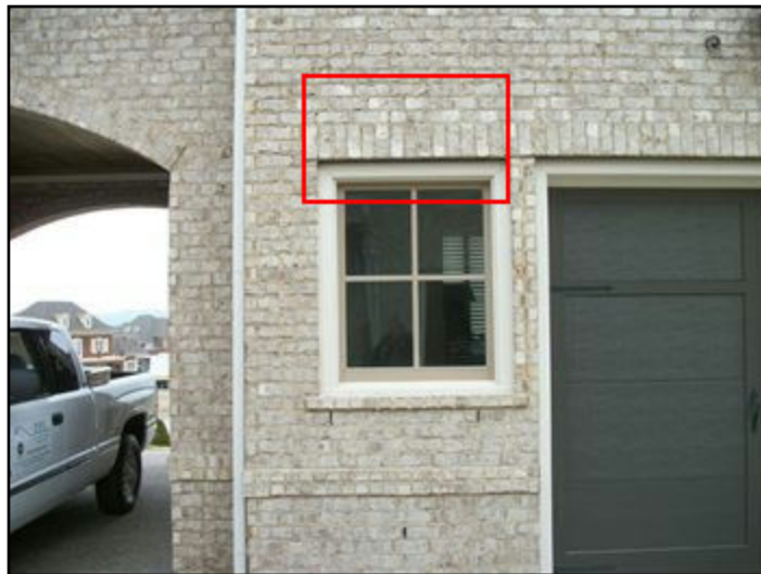
20. Missing weep holes
