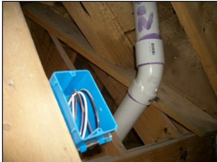
35. Wires not properly terminated
