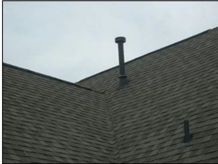
14. Peeling paint on flue
