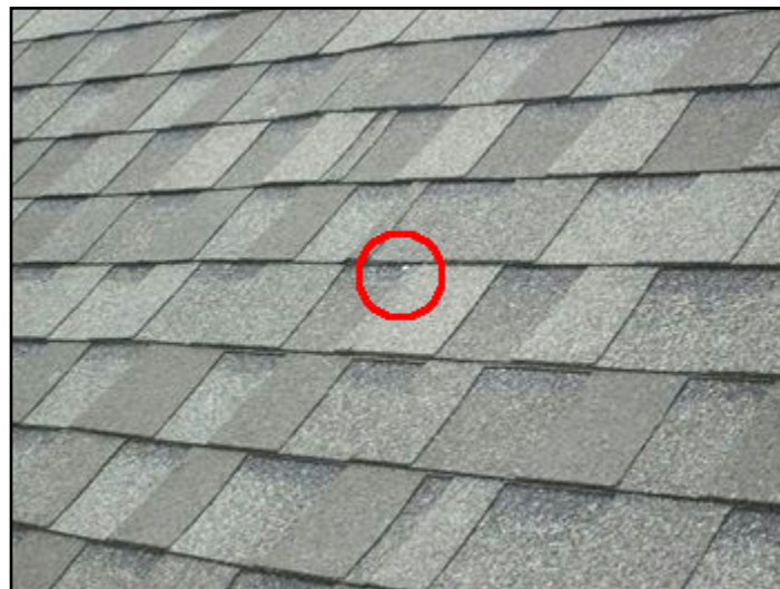
12. Exposed fastener @ garage
