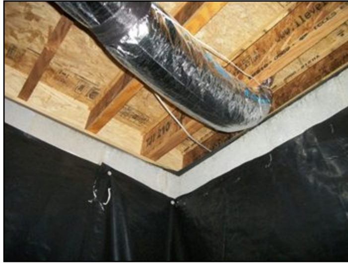
40. Missing rim insulation
