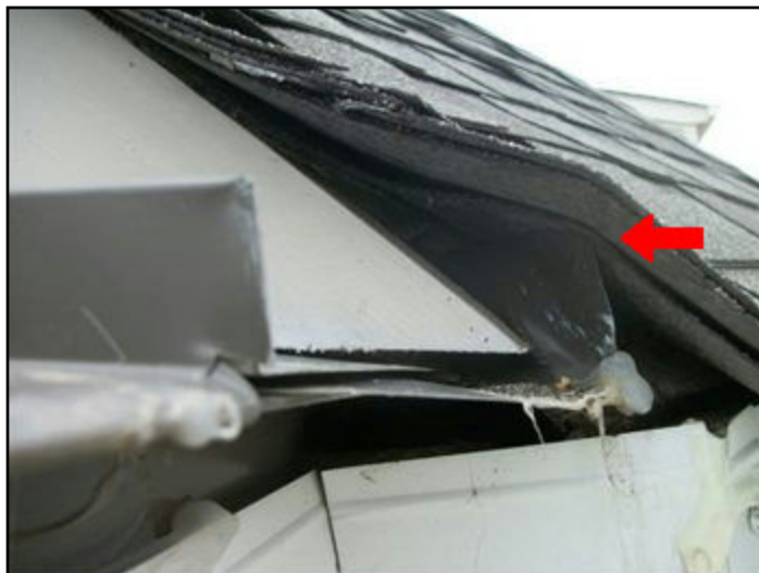
3. Flashing is tearing a shingle
