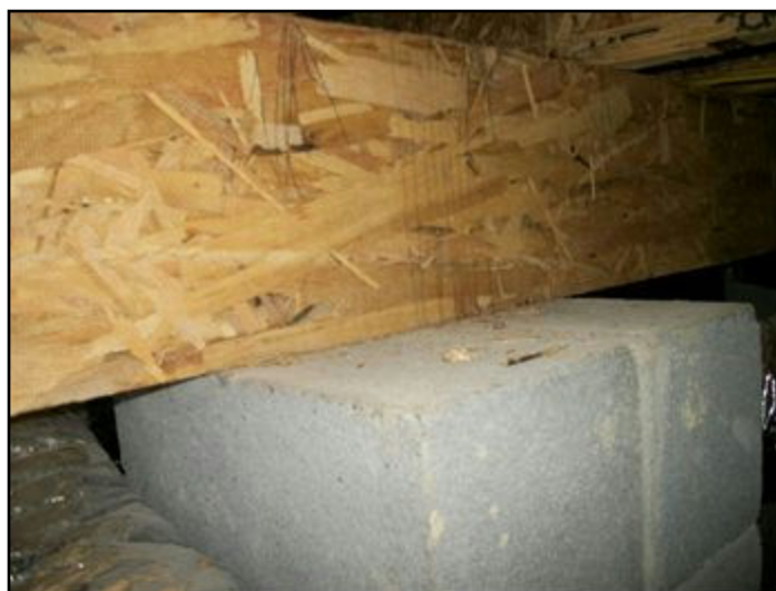
24. Missing vapor barrier
