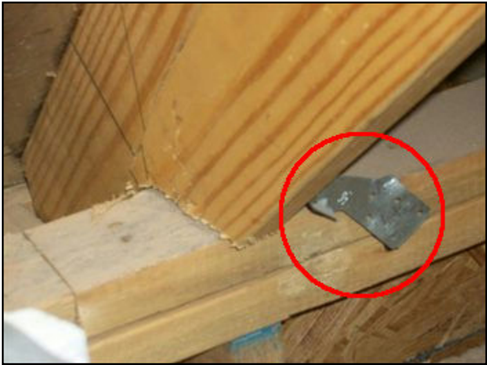
32. Loose tie-down bracket
