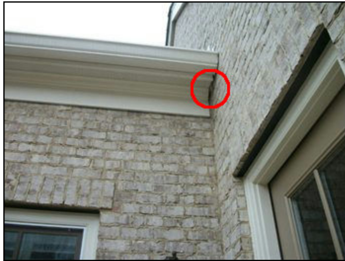
15. Gap in soffit
