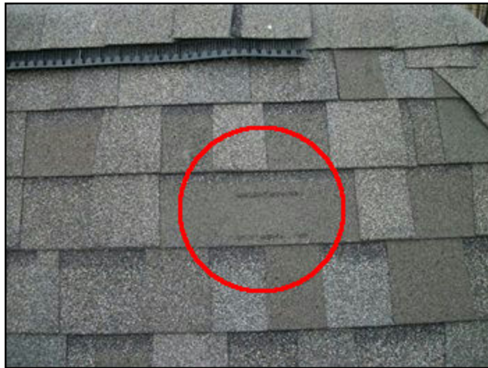
5. Laminated tab is missing
