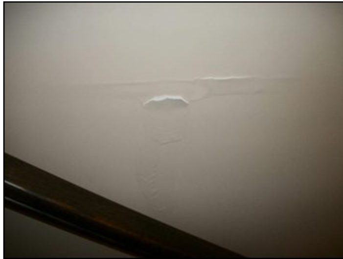
44. Possible water damage
