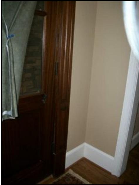
45. Gaps in trim
