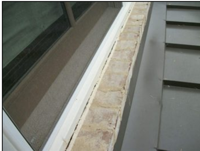
21. Gaps in caulking
