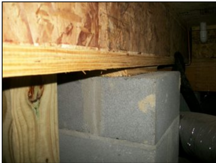
23. Missing vapor barrier
