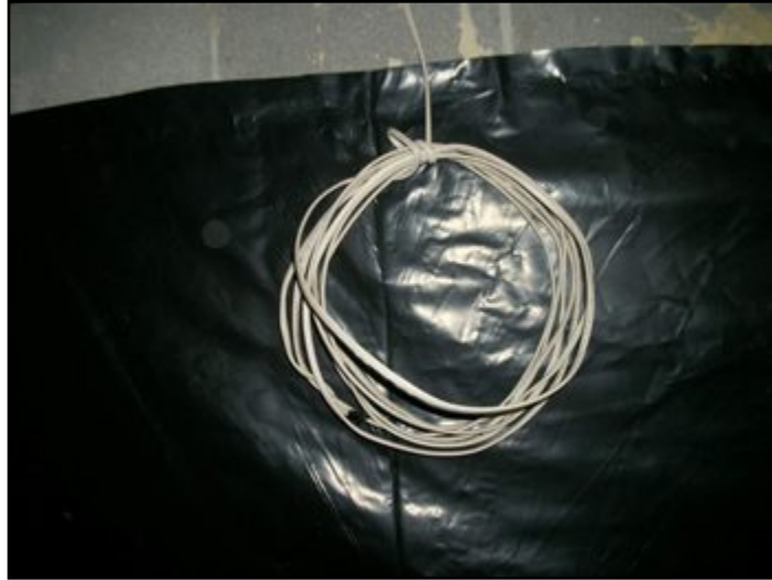
34. Wire not properly terminated
