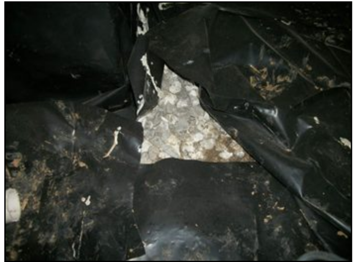
38. Gap in vapor barrier
