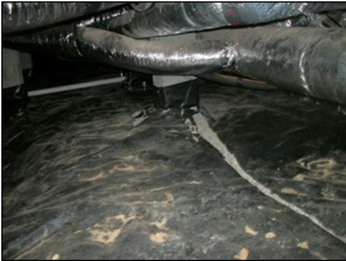
37. Gaps in vapor barrier
