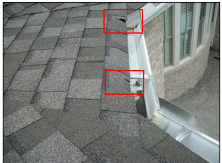
7. Minor shingle damage
