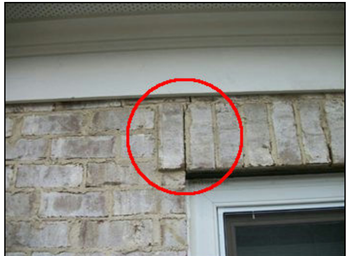
19. Crack in mortar joint
