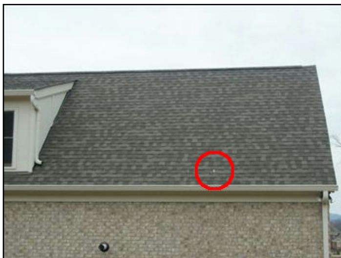
4. Debris under a shingle
