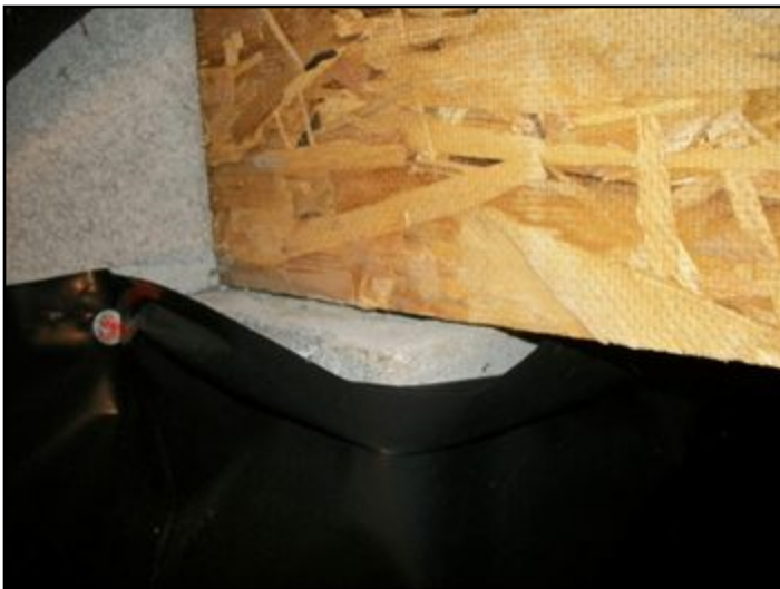
22. Missing vapor barrier
