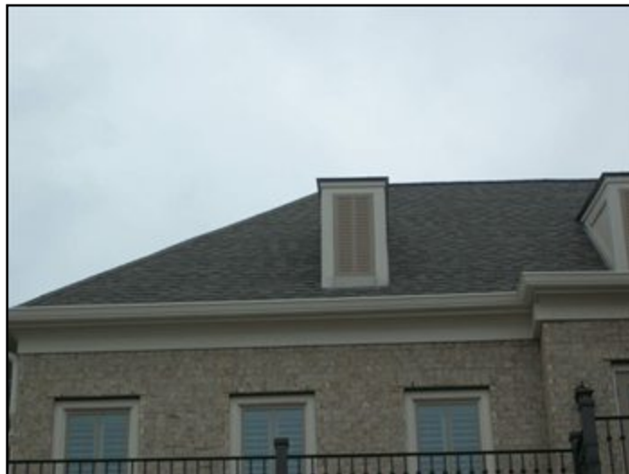
16. Trim needs painting
