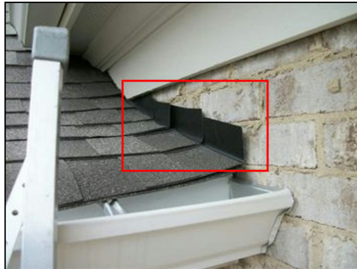
13. No counter flashing
