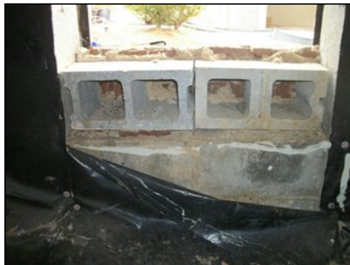
39. Vapor barrier pulled loose from wall
